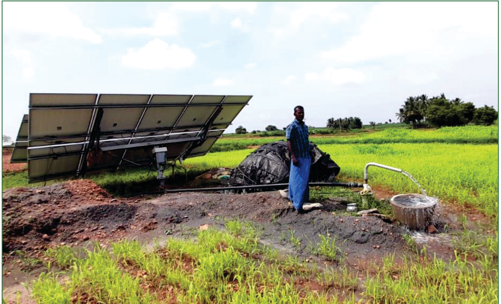
Picture 3 : Solar water pumps used for irrigation
